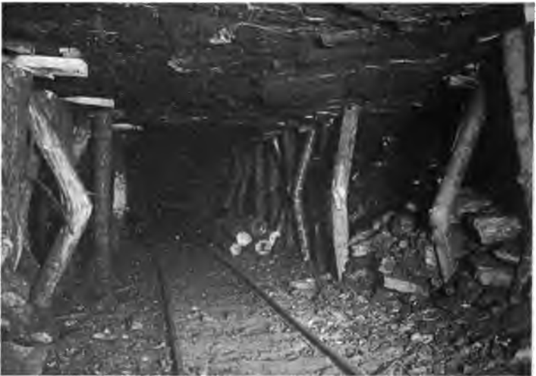
Fig. 11. Timber Broken by Squeeze, Anthracite Coal Mine, Scranton, Pa.
